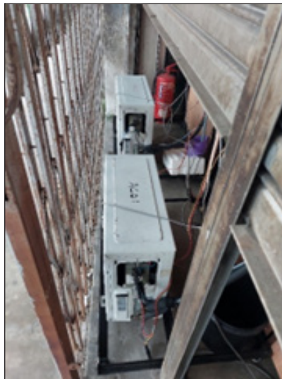
Figure 4. Complete outdoor compression condenser unit setup with measurement gadget
